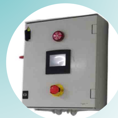
Degassing control box
